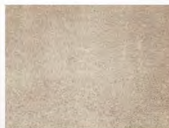
Condition C Blasted to Sa3
