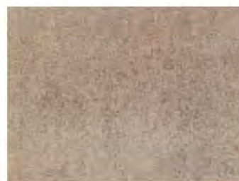
Condition C Blasted to Sa2.5
