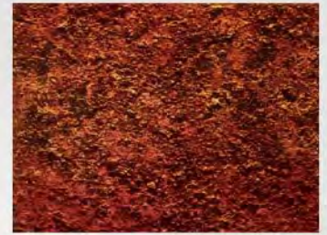
Condition D Unblasted
